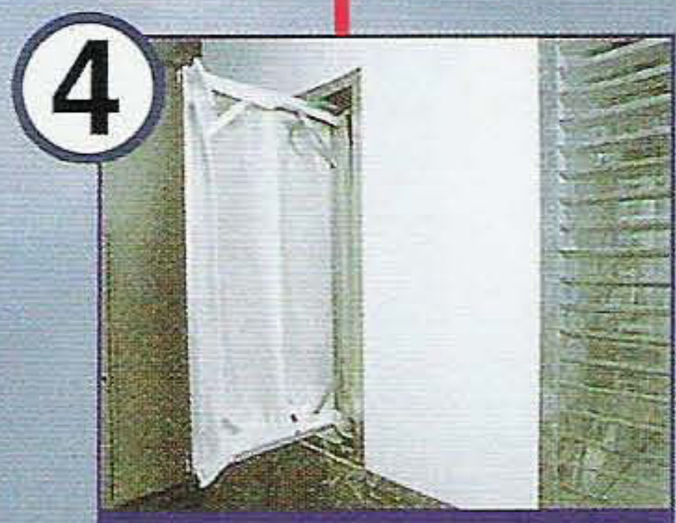
4 THE SECOND EXHAUST FILTER
